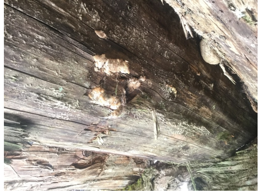
Stringer 2 Fungal Growth
