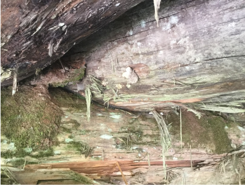
Stringer 4 Fungal Growth
