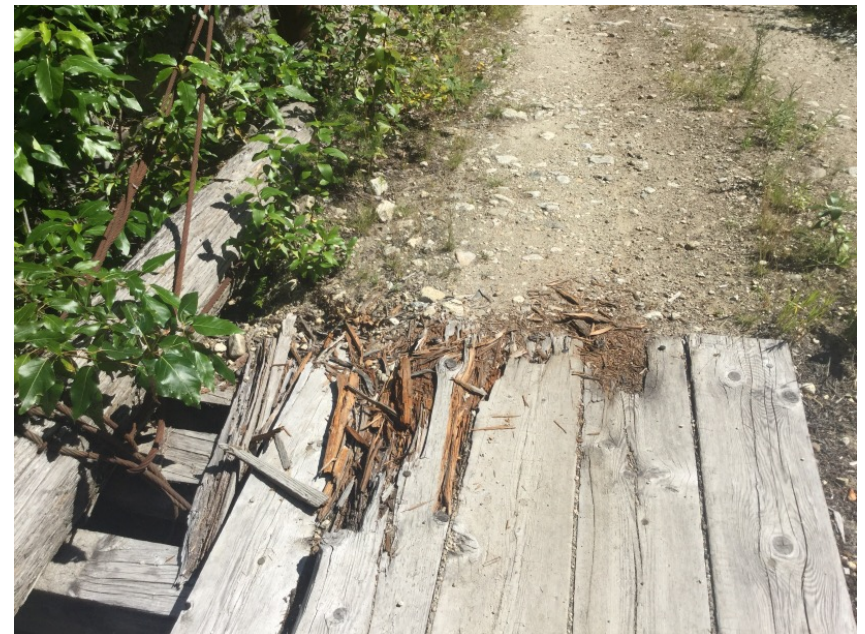
Rotten Deck Planks
