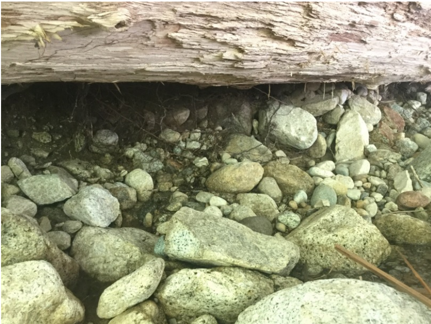
Right Abutment Scour
