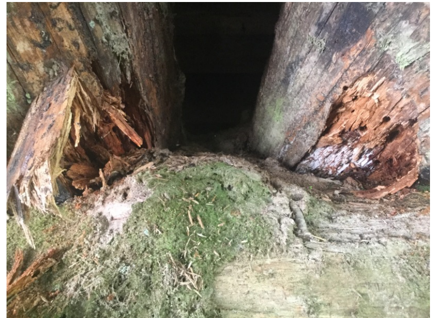
Rot in Stringers 3 & 4
